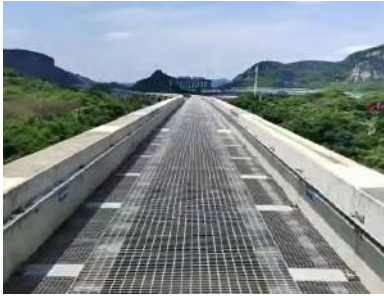
Steel grating platform walkways
