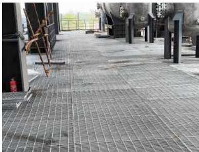
Steel grating platform
