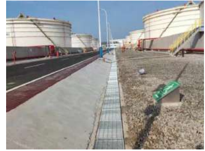
Steel grating trench covers
